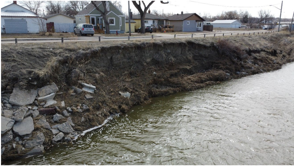
Fig. 1 River Drive Bank Failure
