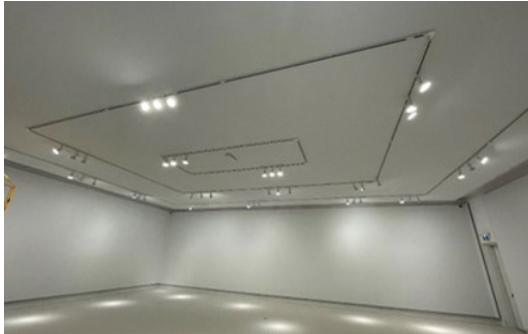
Art Gallery New Ceiling and Lighting
