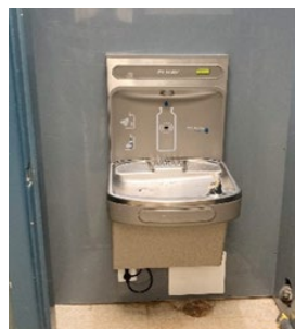
Water Fill Station – LCol Clifton Centre
